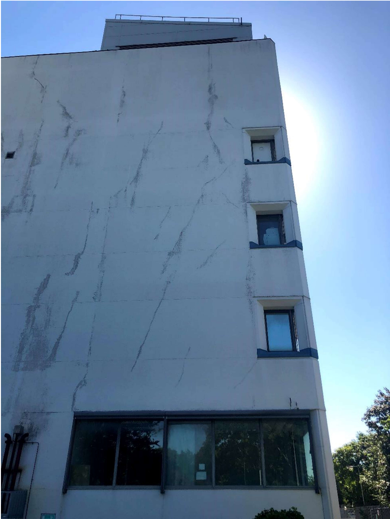
Figure 30. The site is presently derelict, with signs of poor repair throughout.
