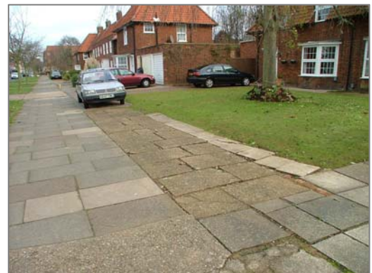
Erosion of grass verges with poor quality paving is exacerbated by parked cars.
