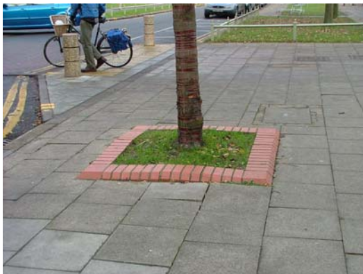
Example of random floorscape treatment in the public realm. Note original guard rails in background.
